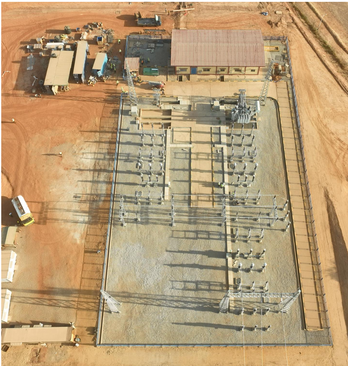
Completed Powerline and Substation – Photo 1
