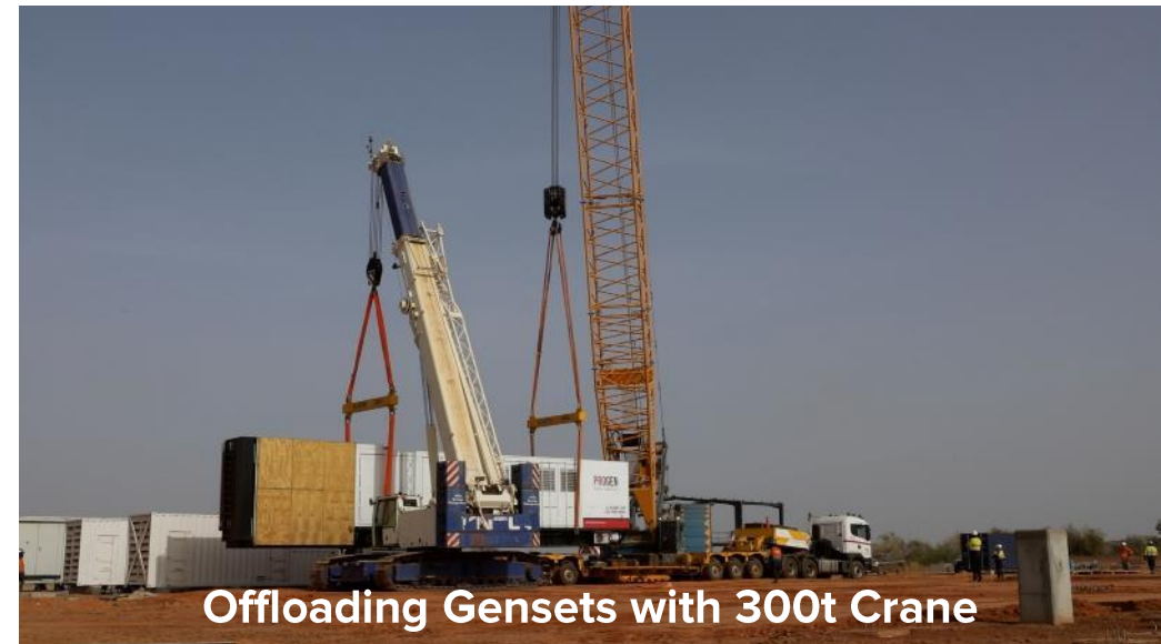
Gensets Arriving on Site
