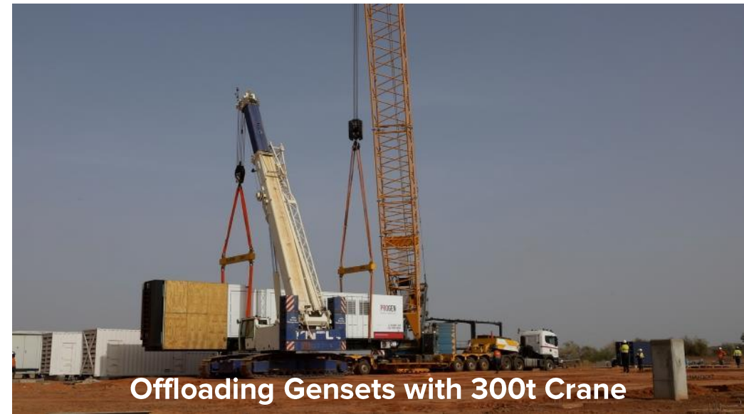
Gensets Arriving on Site
